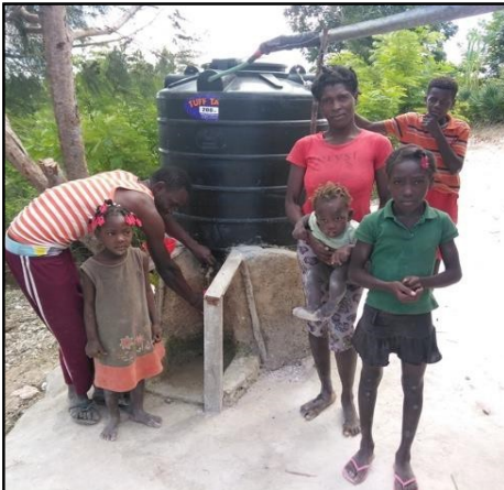
The Fednor Jean family in Nan Mango with their new rainwater catchment system
